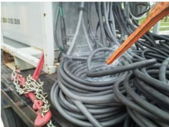
Improper Cable Layout
